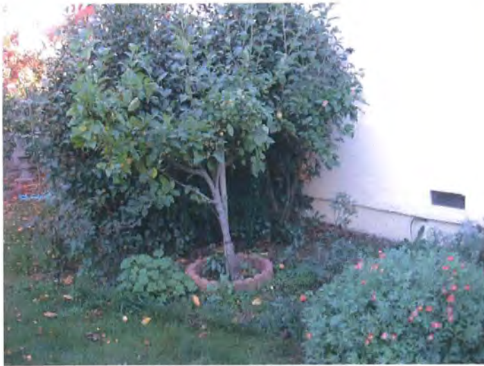
RIGHT VIEW, AIR CONDITIONER IS BEHIND SHRUBS
